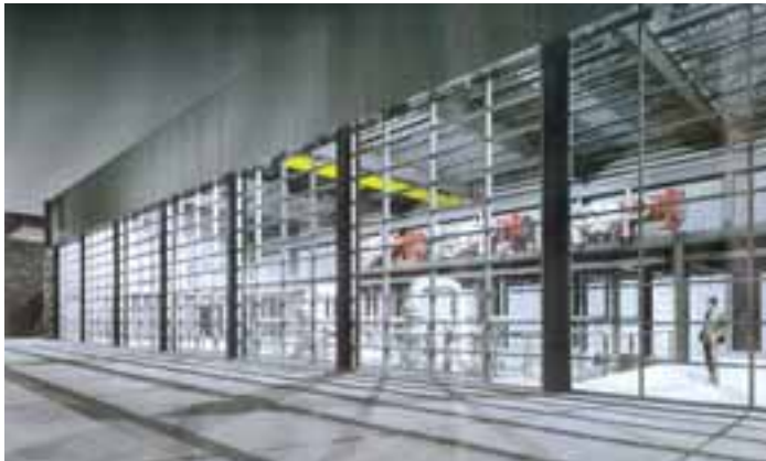
Three HOFIM Sealed units for the Stagecoach Gas Storage project in New York State, USA
